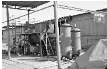
Effluent Treatment Plant
