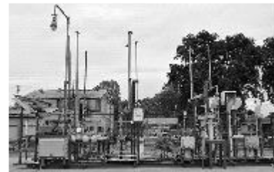
Natural Gas Plant
