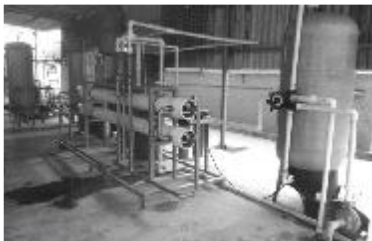
DM Water Plant
